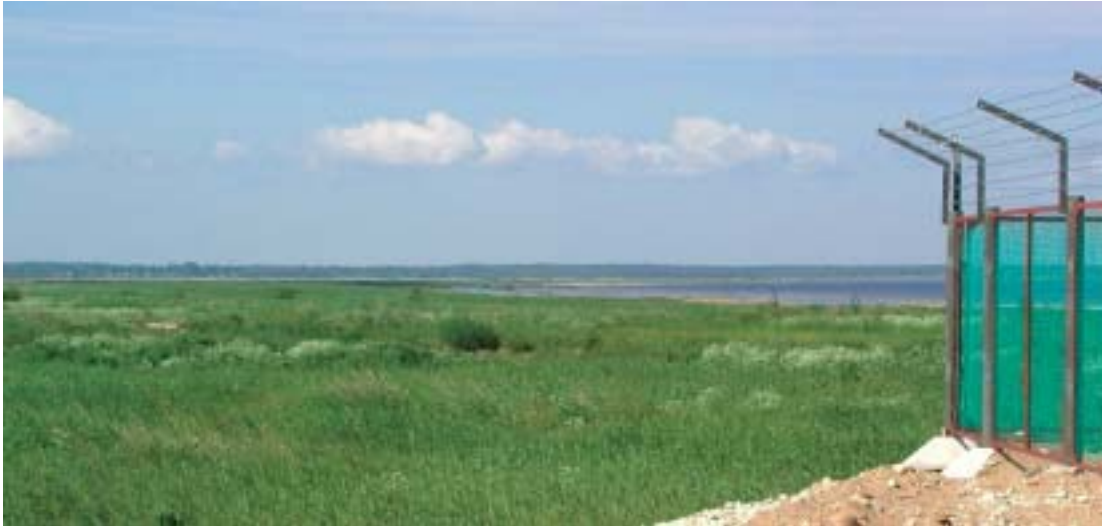
Figure 6 Reed at the construction site of the Multi-purpose Terminal (the fence of the lighthouse is on the right).
